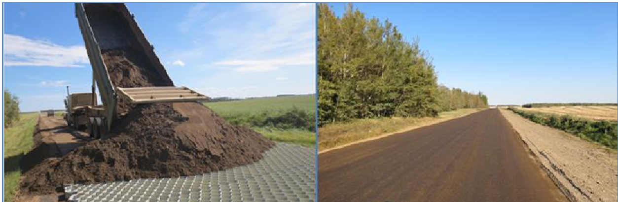
Figure 5: Township road 762 in MD of Smoky River County during a) construction and b) after operation
