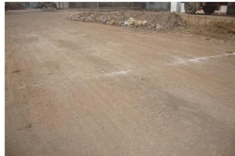
Figure 3. Reinforced Section at Dairy Factory – Level Surface Shown by White Line
