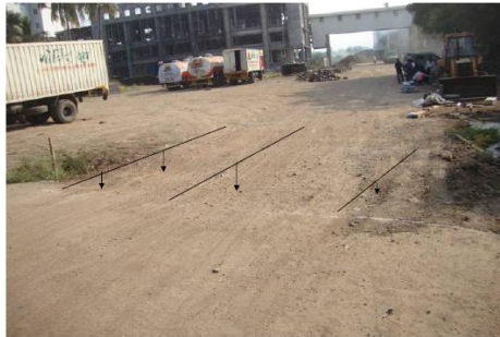
Figure 2. Unreinforced Section at Dairy Factory – Rutting Indicated by Arrows
