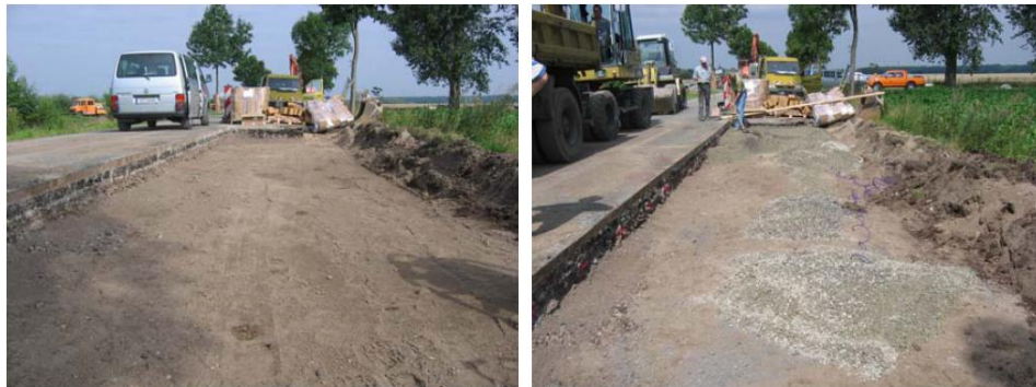
Figure 1: Subgrade (L) and installation of the new gravel base course 0/22 mm (R)
