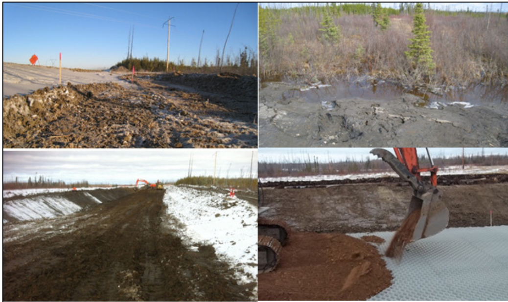
Figure 4: Construction (top left: Frozen muskeg, top right: Water at Ground Level, bottom left: before Installing Neoweb, bottom right: Installed Neoweb)
