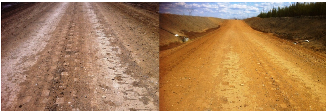
Figure 6: Causeway Surface after 3 Months of Use
